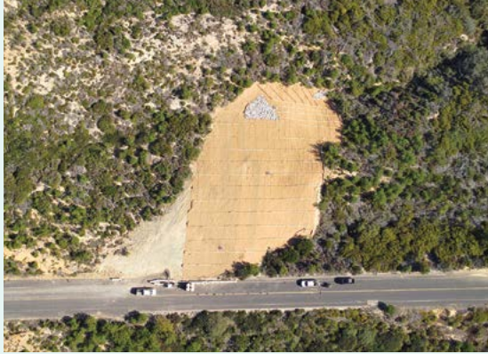
The slide erosion area after the Sealaska Constructors team's restoration work, which was done to control erosion and prevent further damage to the roadway.
